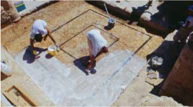
Figure 28. A layer of lime-wash applied to the surface of a mosaic. Trench 2, mosaic M14.
