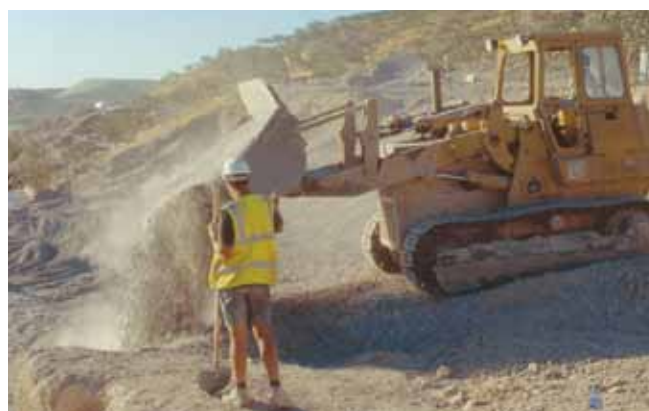
Figure 38. Once the archeological remains are covered, the reburial is completed with gravel and stones.
