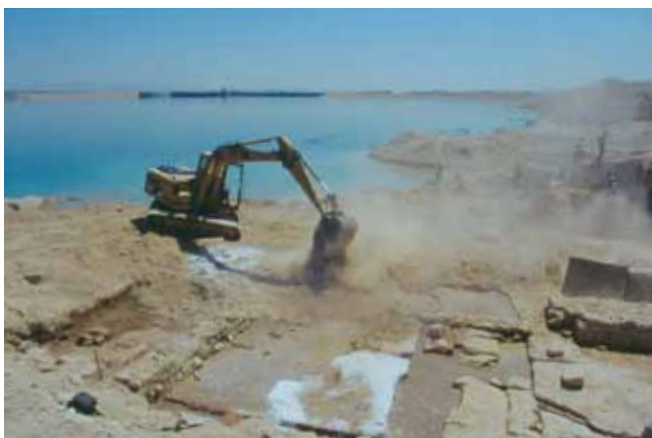
Figure 37. A protective layer of soil is put in direct contact with archaeological features already coated with protective mortar.
